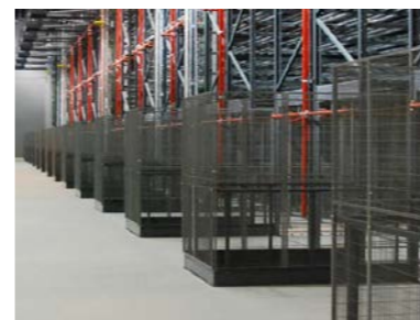
10 TRUCK AISLES The Partitioning System allows warehouse trucks to come through without compromising the safety of personnel or goods.
